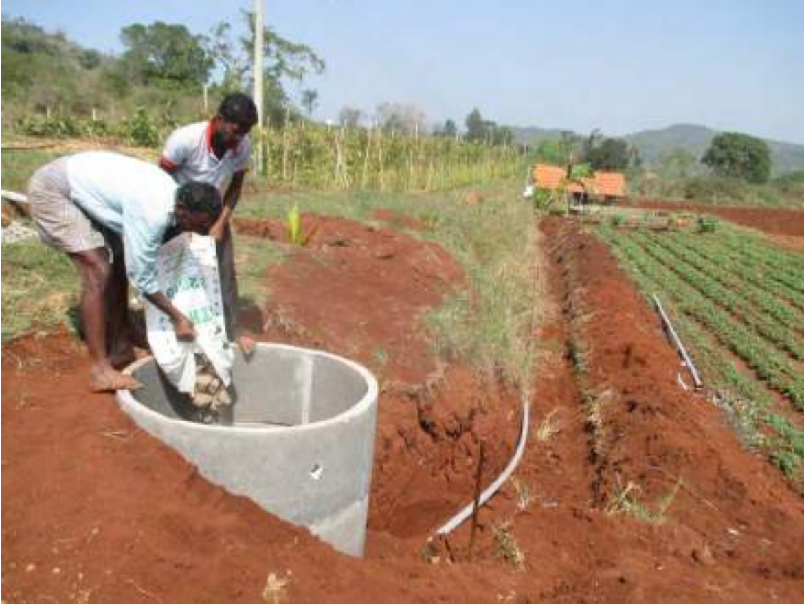
Photo: Well recharge pit fitted with modular cement rings and portable filtration units, channelising surface runoff into the dug well to enhance groundwater recharge.
