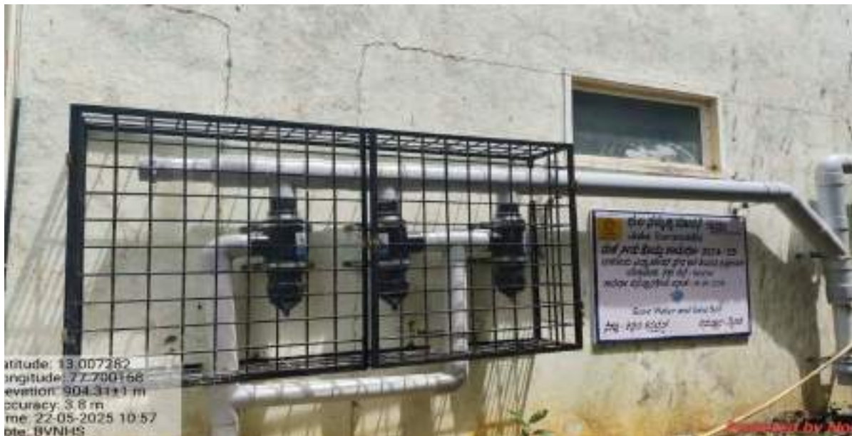
Photo: Rooftop rainwater collection system in a school building, marking the starting point of decentralised rainwater harvesting in an urban institutional setting.
