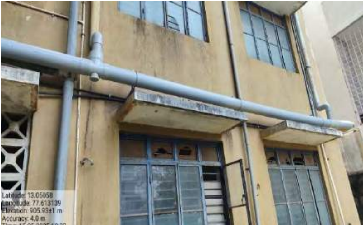
Photo: Rainwater filtration and conveyance system showing gradual increase in pipe diameter from rooftop to underground sump, optimising flow capacity while minimising material costs.
