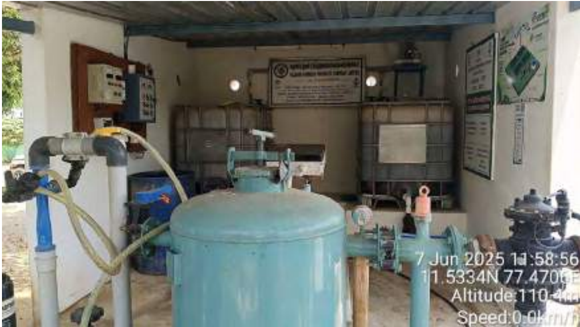
Photo: Central control unit of the automated irrigation system, containing controllers, solenoid valves, pipelines, and fertigation equipment that regulate water and nutrient delivery across the farm.
