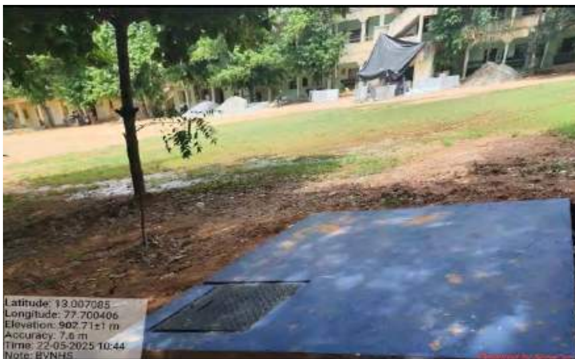
Photo: Underground rainwater storage tank supplying harvested water to an overhead tank, enabling non-potable use such as toilet flushing and reducing dependence on municipal water supply.
